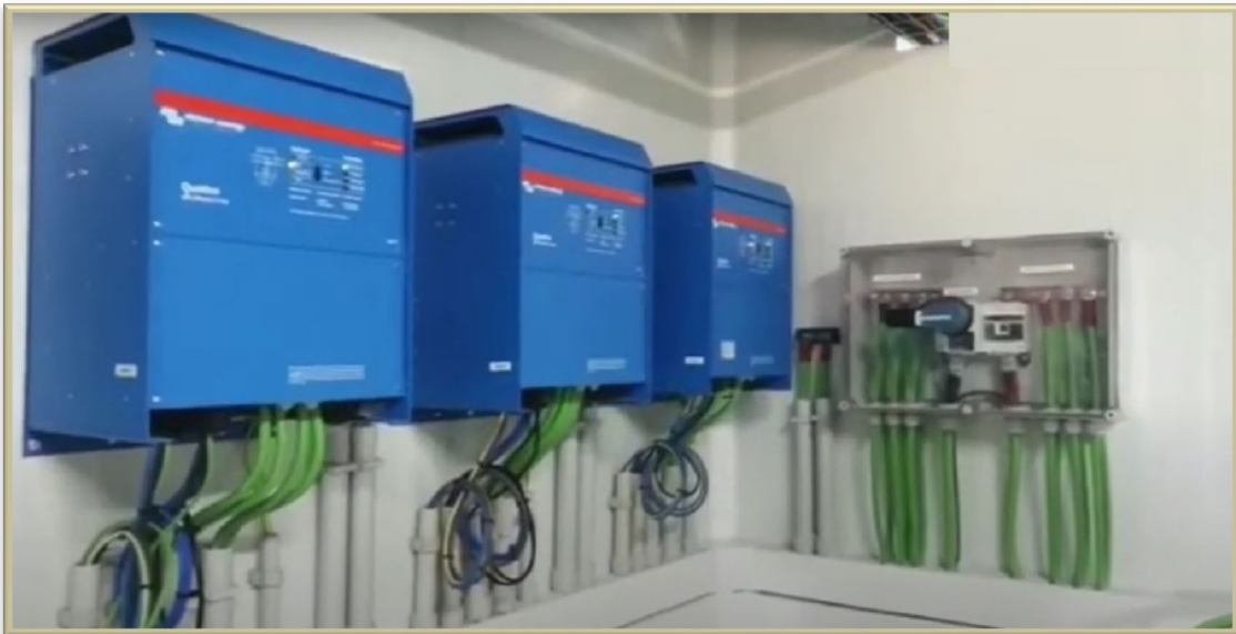
Image 3: Inverters and voltage and voltage regulators
